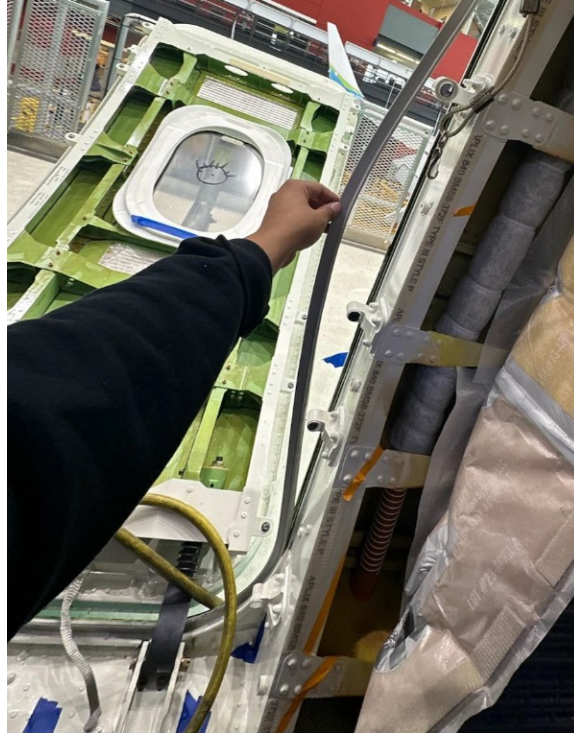
Figure 15. Photo showing the MED plug opened to work on damaged rivets. (Source: Spirit AeroSystems.)
