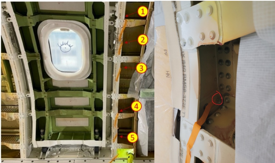
Figure 14. Photo on the left shows the five locations of the damaged rivets. Photo on the right is a close-up of a damaged rivet. (Source: Boeing. Image Copyright © Boeing. Reproduced with permission.)
