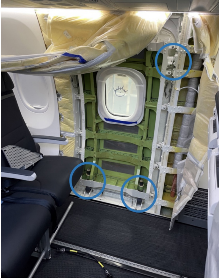
Figure 16. Photo showing the left MED plug immediately before interior restoration and the circles show the three locations without the retaining bolts, two vertical movement arrestor bolts and the forward upper guide track bolt. The aft upper guide track is covered with insulation and cannot be seen in the photo. (Source: Boeing. Image Copyright © Boeing. Reproduced with permission.)
